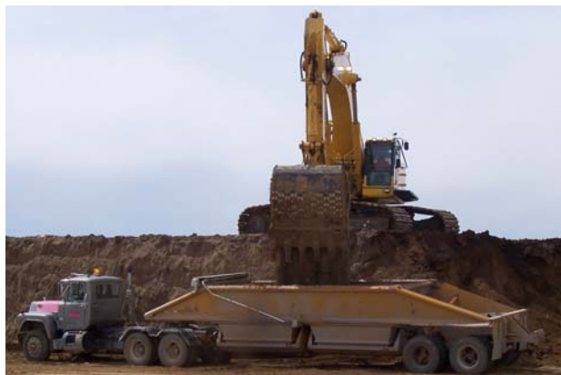
Above: Pink Grading moving dirt from within Phase 1B. Note that the top of the semi is about 11 feet high... WOW!
